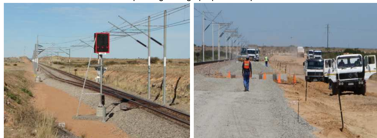
Typical crossing loop – (loop 13 :Kenhardt) left, loop construction in progress (loop 1), right
