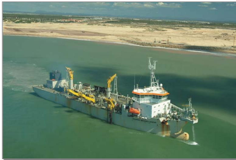
Figure 6.4: Aerial photograph of turbid water generated by dredging during the Phase 1 port construction activities ( photograph supplied by D. Phelp, CSIR ).
